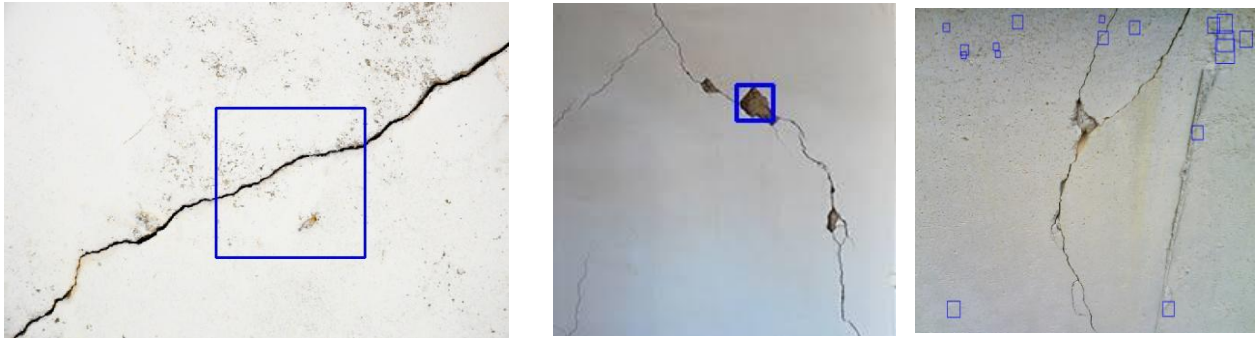
Figure 32 : Detected cracks on Images for stage 12, 10 and 8
